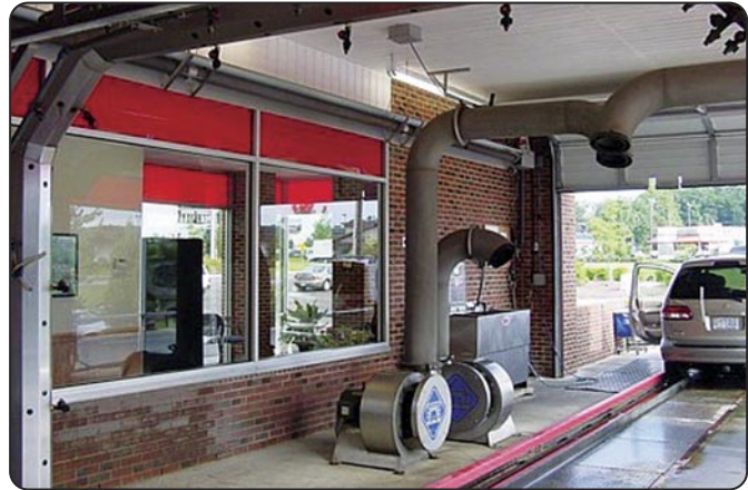
Exit area of an AUTOBELL® tunnel car wash facility
