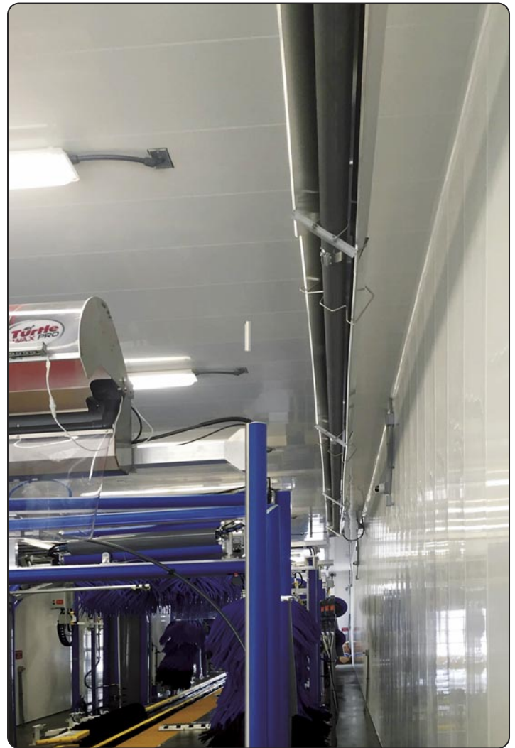
A tunnel wash facility in Baltimore, MD
